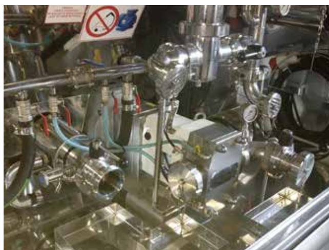
Pumped liquid - transporting syrups, chocolate, etc. Pump - LPX80-1 installed on a truck cistern
